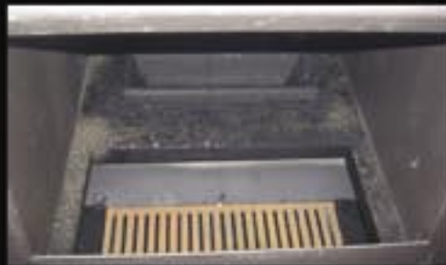
Photo ashes removal
